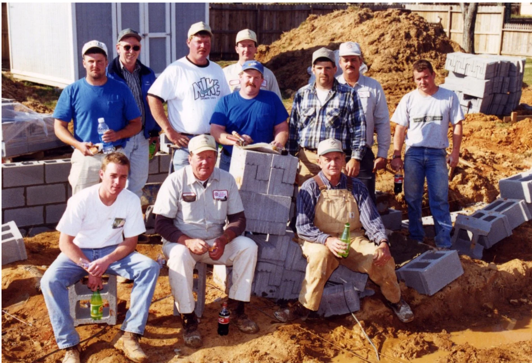
A Western Carolina Chapter workday installing a foundation as a fundraiser in March of 1999.
